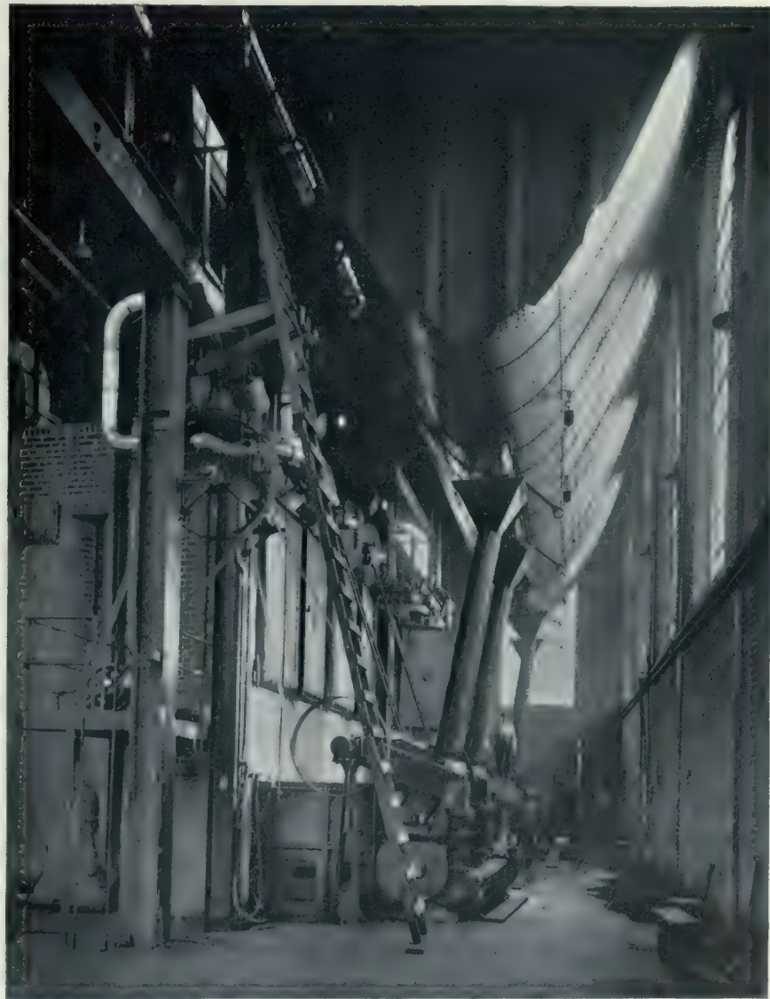
BOILER ROOM, SHOWING MECHANICAL STOKERS.
