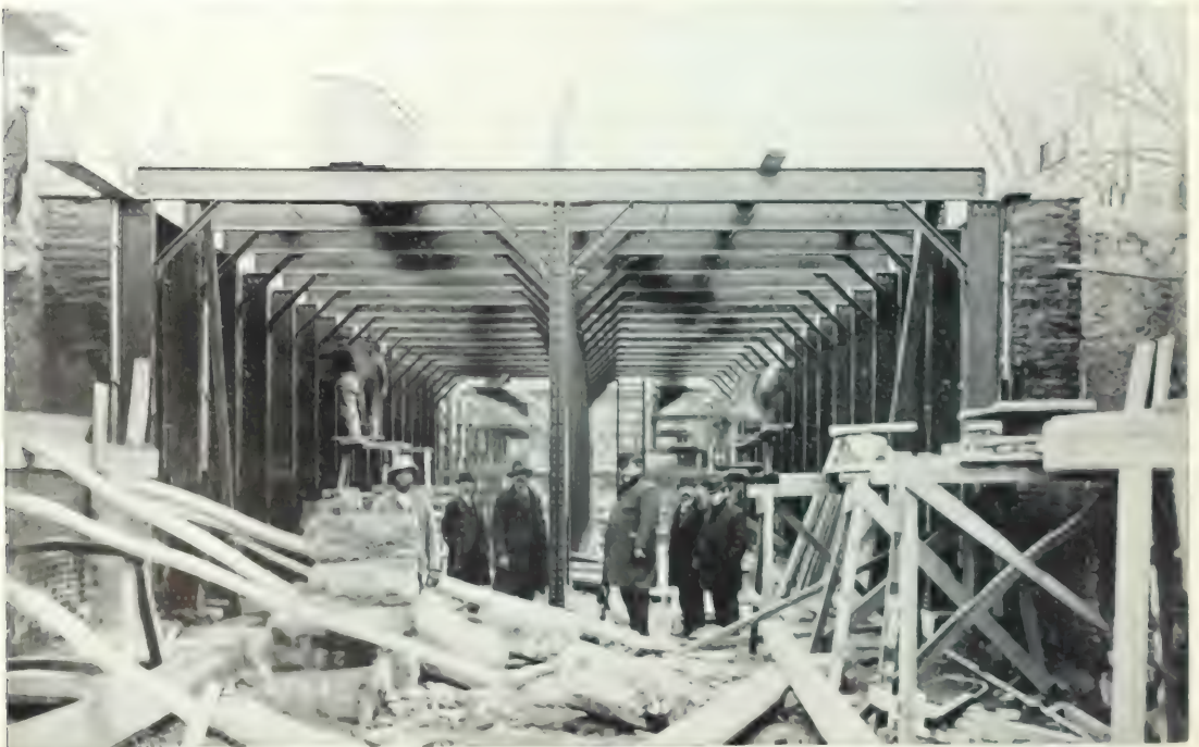
VIEWS OF THE NEW SUBWAY IN NEW YORK CITY Taken in the quality where sand rock has been pierced by means of blasting.
