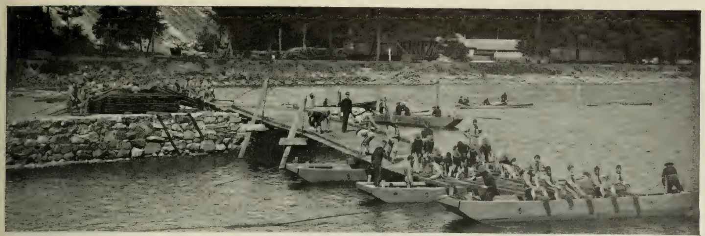
PONTOON BRIDGE BUILDING Binding the timbers at the beginning of the bridge
