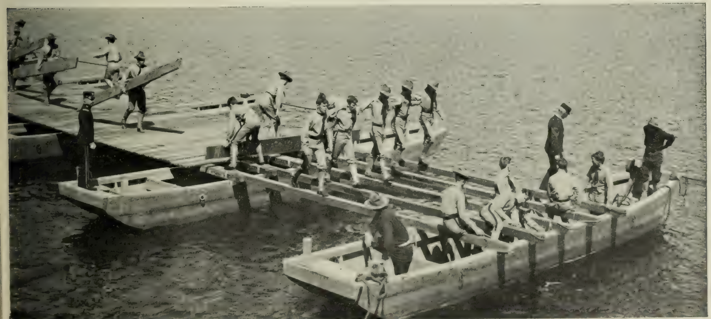
PONTOON BRIDGE BUILDING Laying crosspieces and making ready for the next pontoon and the long timbers
