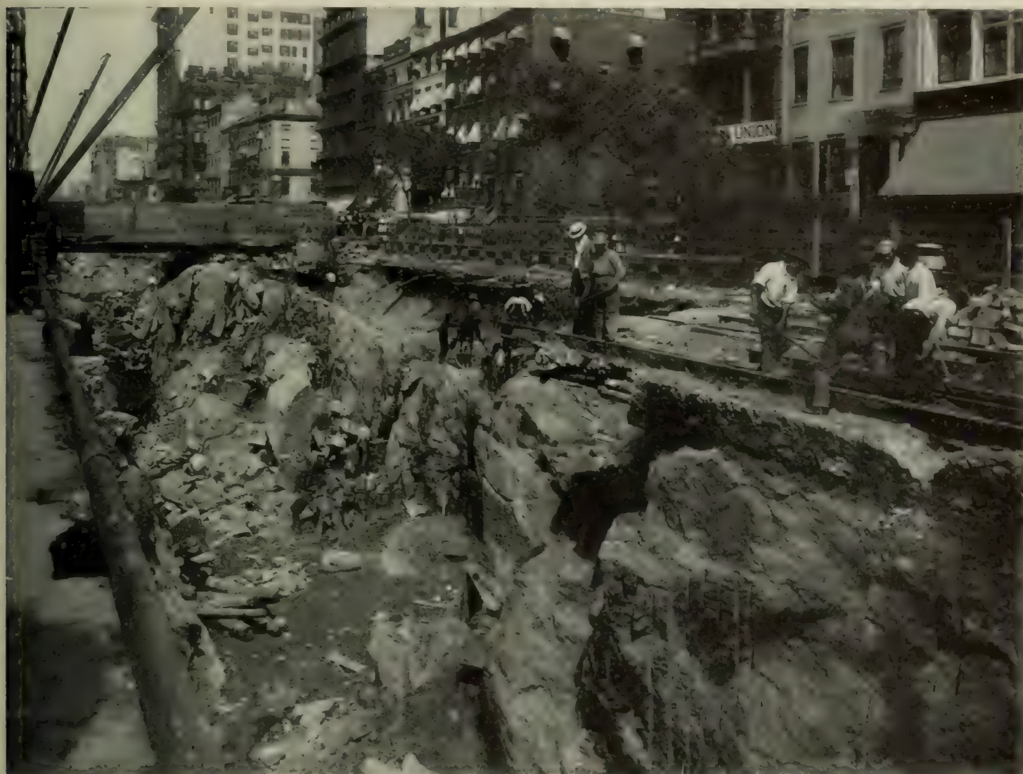
UNION SQUARE WHEN THE WEST HALF OF THE TRENCH HAD REACHED ITS DEPTH
