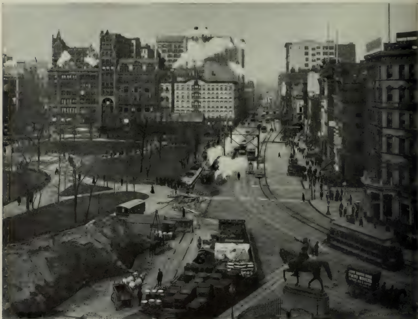
UNION SQUARE AS THE WORK WAS BEGINNING ON THE WEST SIDE OF FOURTH AVENUE The first of five pictures taken at the same place showing the "cut-and-cover" method of building the greater part of the subway
