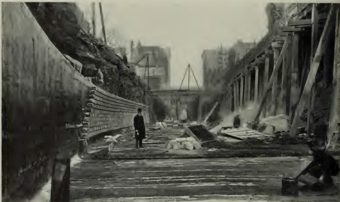
FINISHING THE WEST HALF OF THE TRENCH AT UNION SQUARE—THE METHOD OF WATERPROOFING THE BOTTOM AND SIDES SHOWN
