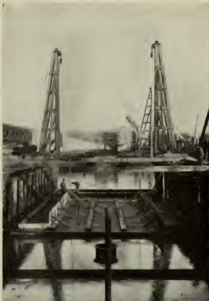
A NEW ENGINEERING FEAT — SINKING SECTIONS OF THE SUBWAY TO MAKE A TUNNEL UNDER THE HARLEM RIVER
