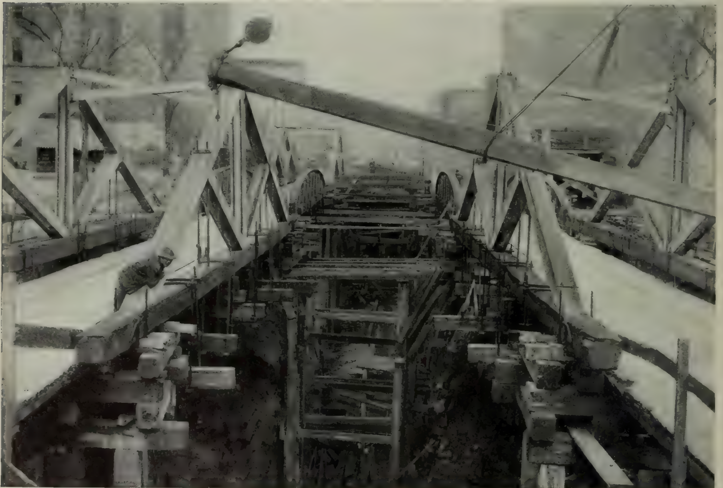
HOW THE SURFACE TRACKS WERE SUPPORTED WHEN BOTH SIDES OF THE STREET WERE UNDERMINED —THE TWO FORMS OF BRIDGE SHOWN
