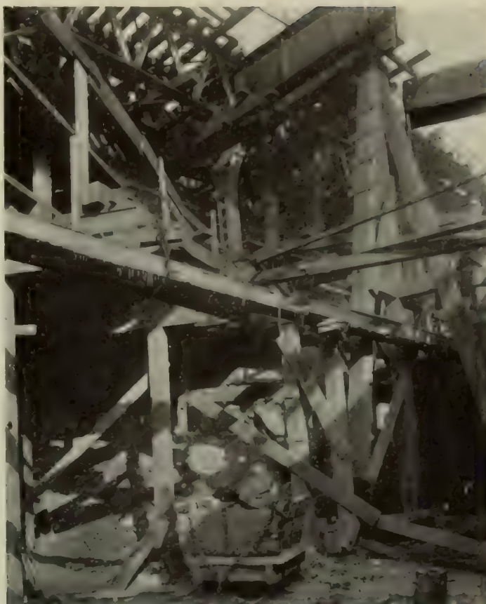
WHERE THE ELEVATED RAILWAY HAD TO BE SUPPORTED WHILE THE SUBWAY RAN BENEATH
