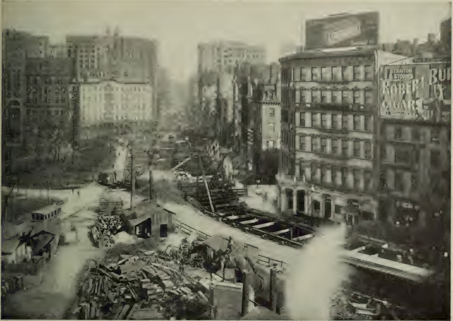
THE WEST HALF OF THE SUBWAY AT UNION SQUARE FINISHED AND COVERED AND THE EAST HALF UNDER WAY
