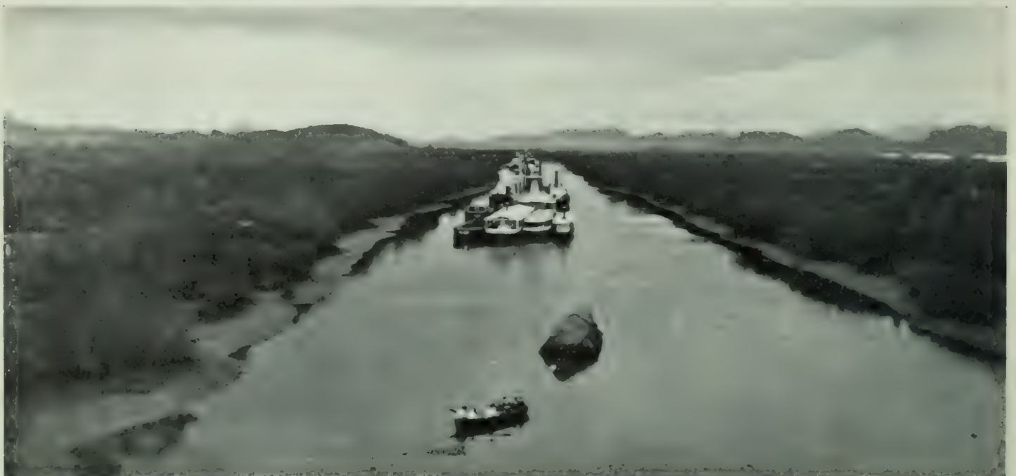
DEEPENING THE RIO GRANDE RIVER NEAR PANAMA Showing the flat country through which a section of the canal goes
