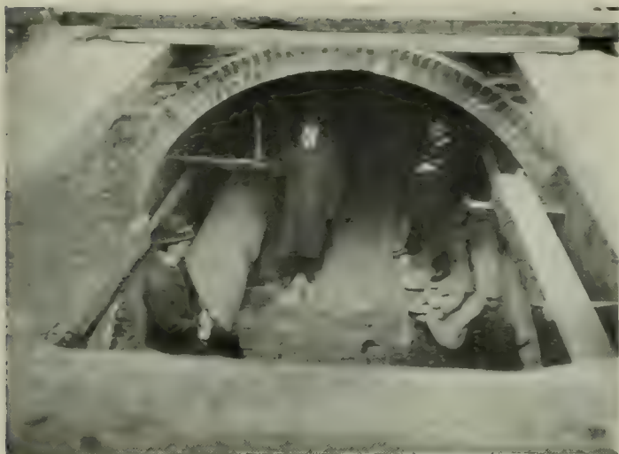
GALLERY FOR PIPES AND WIRES BENEATH THE STRAND
