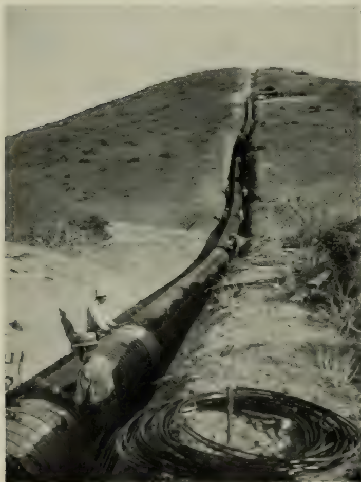
PUTTING THE IRON BANDS ABOUT THE WATER-PIPE LEADING DOWN THE MOUNTAINS The reservoir is far beyond the top, up another mountain
