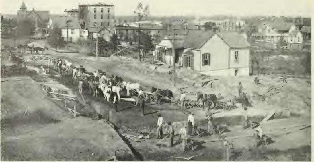
THE STUDENTS DIGGING THE FOUNDATIONS FOR THE C. P. HUNTINGTON MEMORIAL BUILDING
