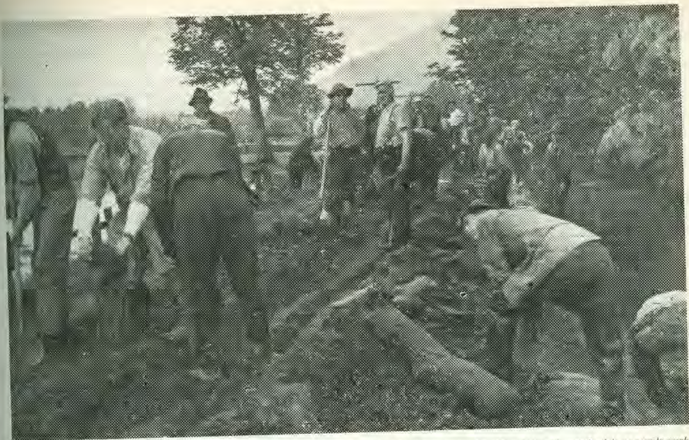
Tuesday, June 1, 1948. The 1948 Flood. Crews work day and night to build up Rosedale dyke. A continuous line of trucks jarred over the dyke to supply workmen with gravel for sandbags.
