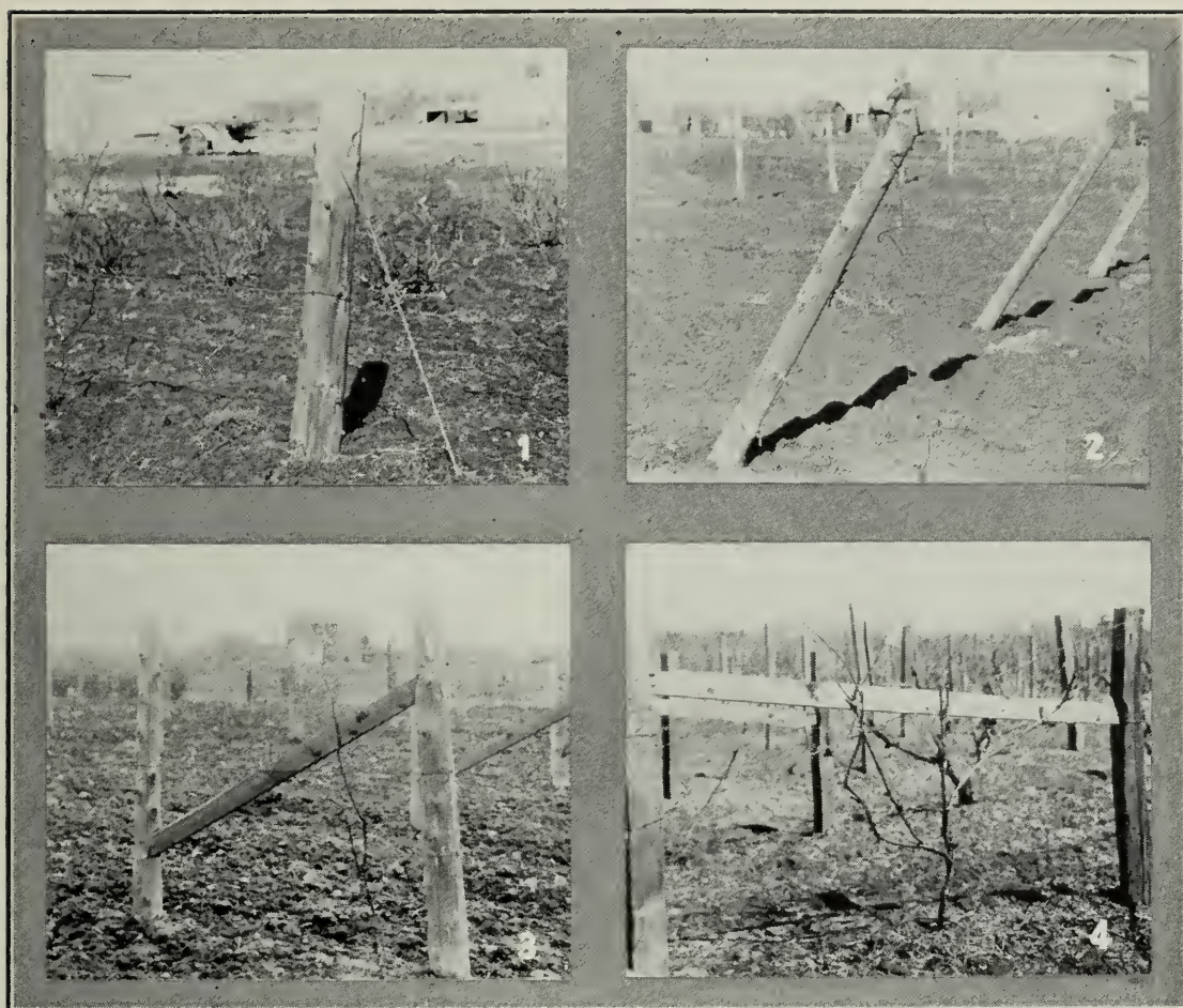
(Fig. 5) Four methods of bracing the end-posts. (1) Guy wire on straight end-post. (2) Guy wire on slanting end-post. (3) Short scantling brace. (4) Long scantling brace between end-post and special second post. Notice the guy wire in each case. Method No. 3 is to be preferred, but is the most expensive.
