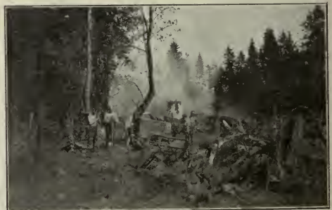
H EAVY work clearing H. B. C. land on Vancouver Island which will be used for a golf course by Victoria residents next summer.
